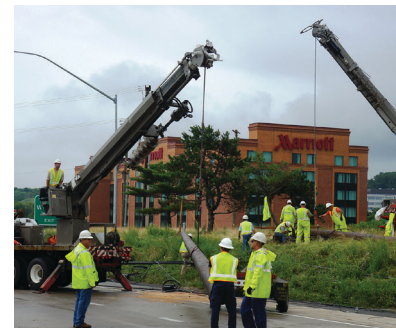
Fire Co. assisted with downed power lines and poles.
