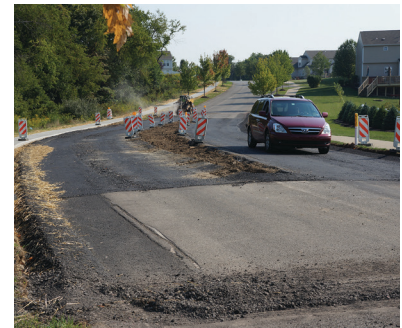
Roadway resurfacing is a fact of life in a busy, growing community.
